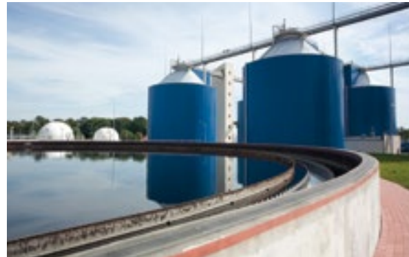
WASTE WATER FACILITIES
