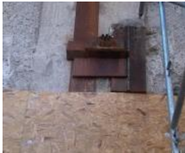
Tie-back (anchoring) of the retaining wall: Not a uniform and continuous substrate, or requires a temporary recess for tie-back.
