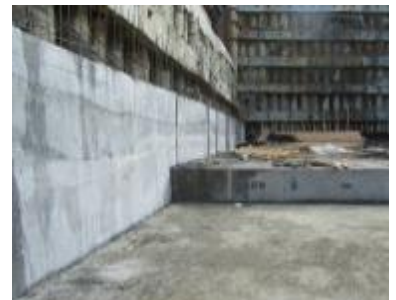
Piled retaining wall with anchors: The uneven substrate with additional levelling/facing concrete/mortar.
