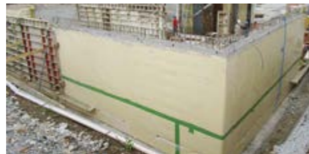
Open excavation with SikaProof®-A – after removing the formwork the anchor penetrations have to be sealed.
