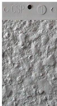
CSP-7: Heavy Abrasive Blast
