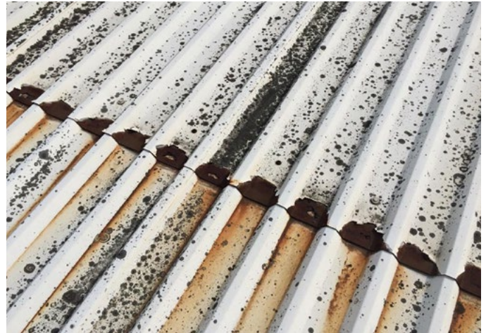
Corroded roof sheet
