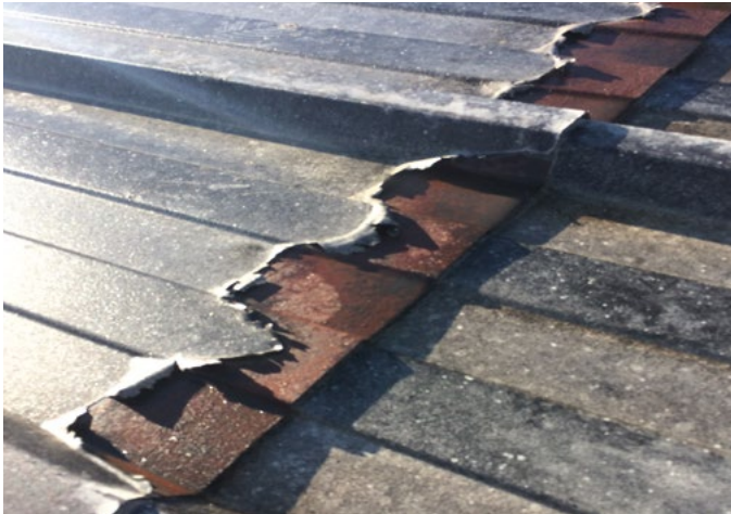
Corroded roof sheet
