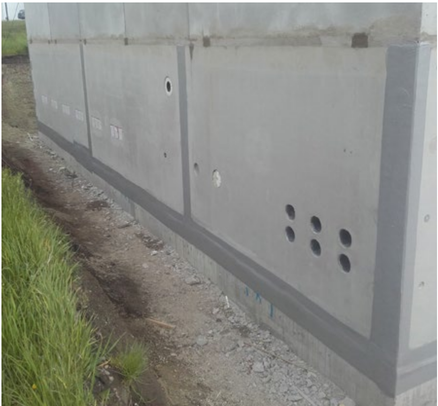
Sealing of construction joints based on the example of a precast basement
