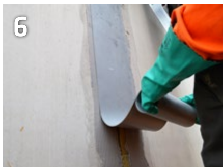
Lay the 2 mm jointing tape into the fresh adhesive layer near an expansion joint
