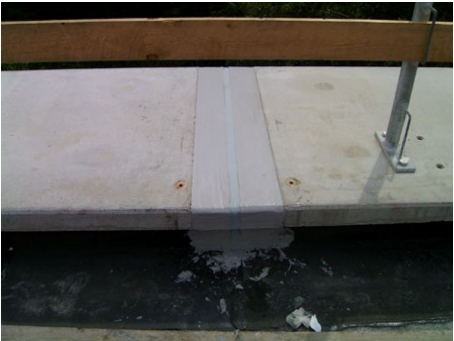
This configuration can be used for waterproofing on bridge constructions and complies with the specifications of the BAST standard drawing FUG 4 sheet 2.
