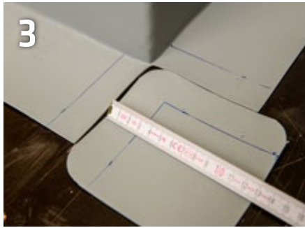
3 Prepare an additional fitting piece taking into consideration the overlap of 30 mm. Round the corners with scissors and mark the overlap area on both sides.
