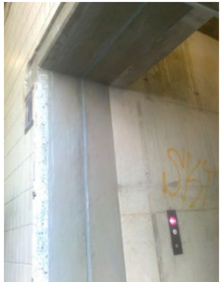
Renovation of an expansion joint - in this case a supporting structure by means of drag plate flashing is required.
