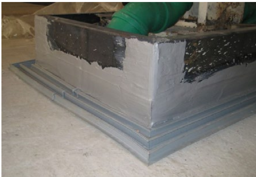
Connection of a new base plate to steel supports by sealing with a DFT waterbar profile
