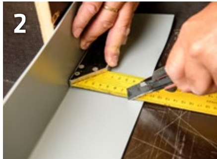
2 Cut the jointing tapes up to the corner and lay around the corner.
