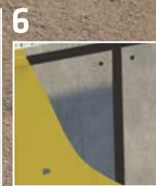
Leaking Compartment Membrane System
