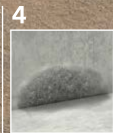
Leaking Areas of Voids i.e. Honeycombing
