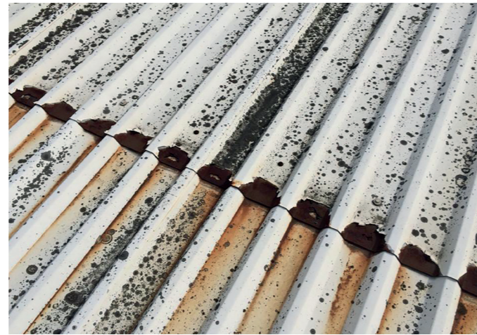
Corroded roof sheet
