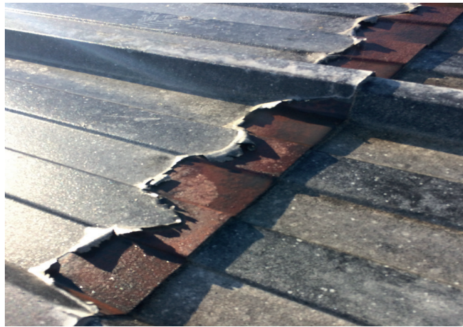
Corroded roof sheet
