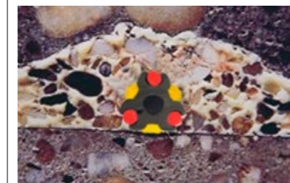
Neoprene strips (red) are compressed under injection pressure, injection material can penetrate into the joint and structure (Phase 2).
