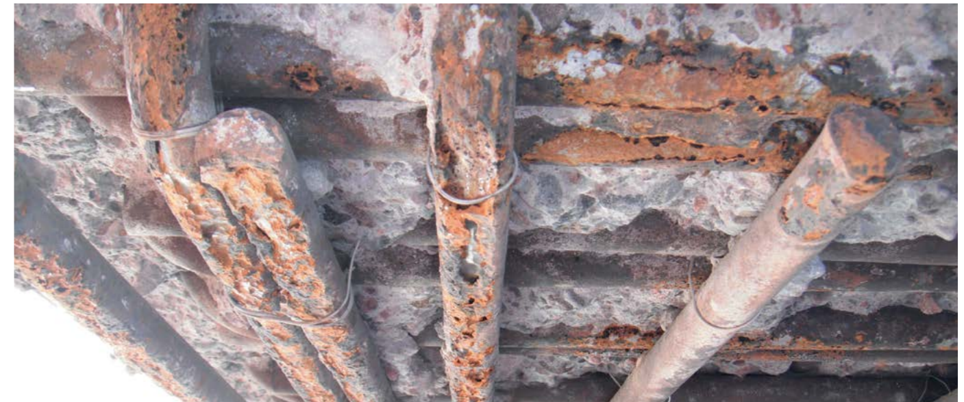
Figure 3. The photo shows exposed rusting reinforcement in a concrete slab that has lost significant section due to pitting corrosion
